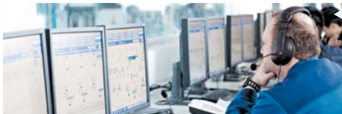
Control and monitoring systems for Hebei Yongxin Paper's packaging paper machine.
